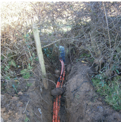
Several multicore ducts going under a fence.
