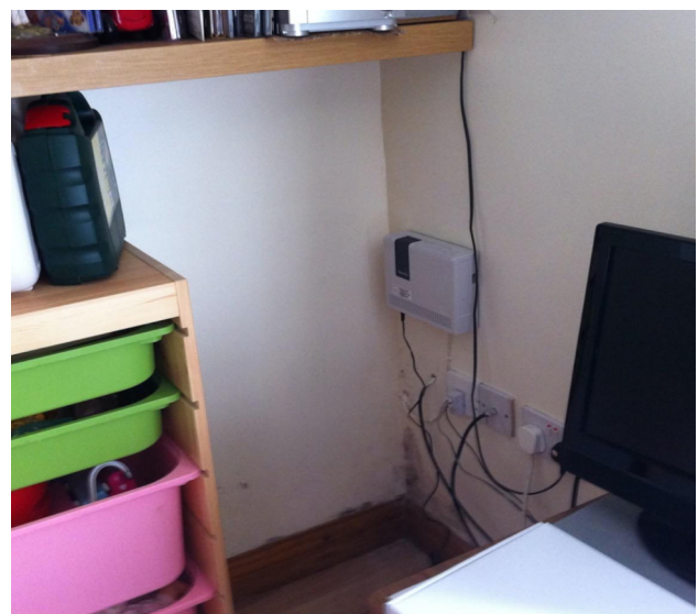
The router in position on the FTU.
