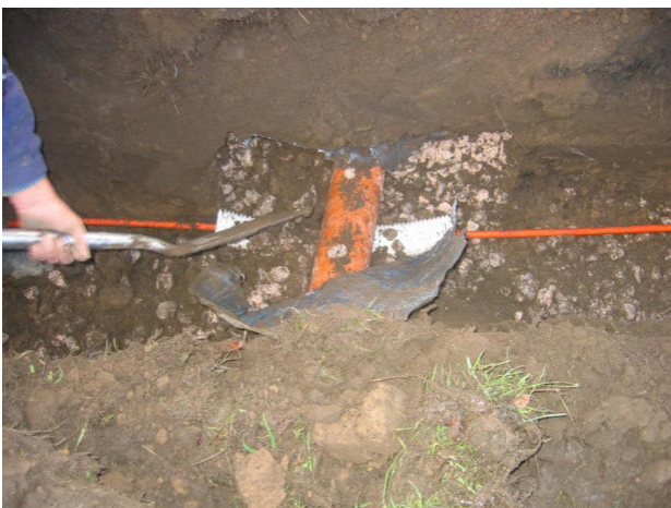
Duct going under a drain.
