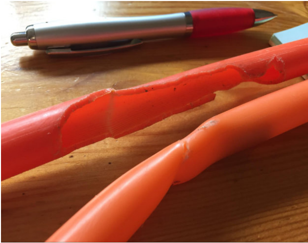
The damaged duct caused by rodents.
